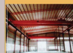
Electric Hoist Bridge Crane
